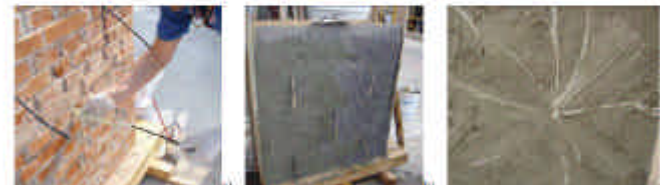
Figure 1. Application of the strengthening layer on the panel PR_G1: (a) Location of the glass fiber mesh; (b) Positioning of the mesh; (c) Anchoring of the connectors.
