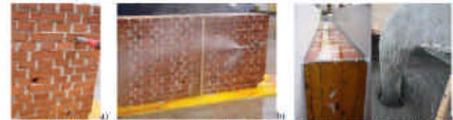
Figure 2. Application of the strengthening layer on the panel P_RT1: (a) Location of five through holes; (b) Hydro cleaning of the surface; (c) Realization of the moulds casting.
